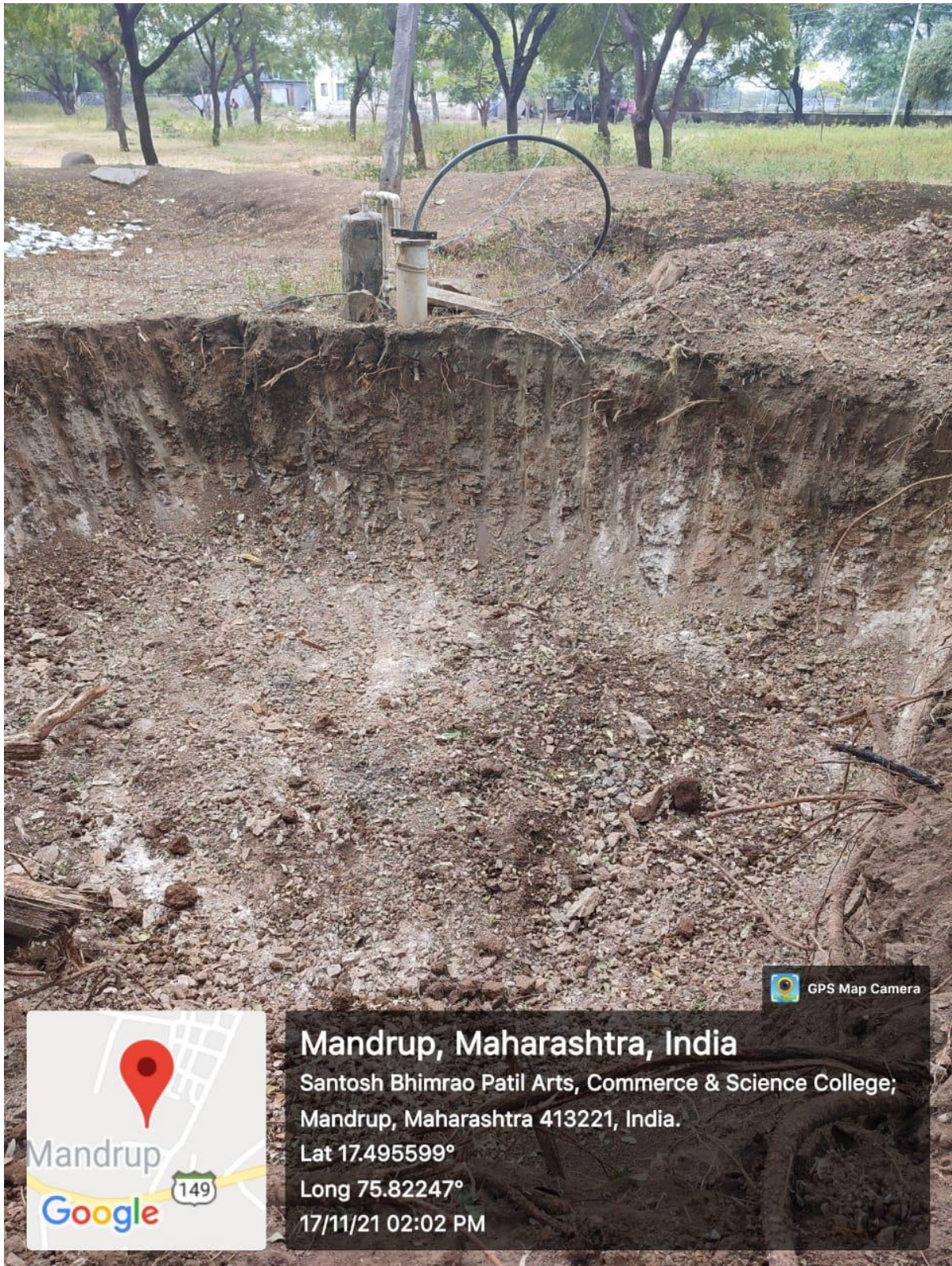
Borewell recharge system
