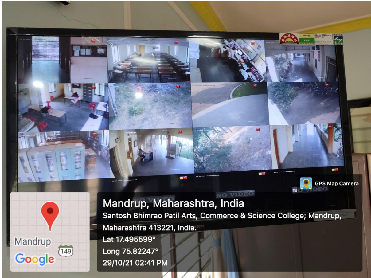
Common CCTV Control Unit
